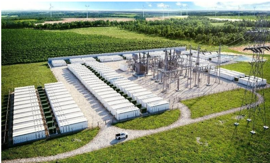
Example BESS site
